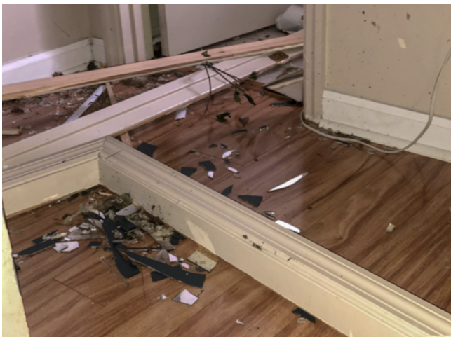
A mirror fell from the wall of the bathroom, along with the door frame.
